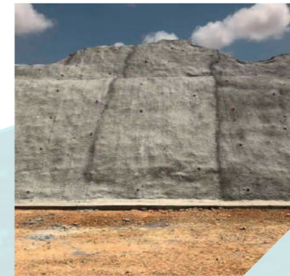
Duqm Gas Supply Station
